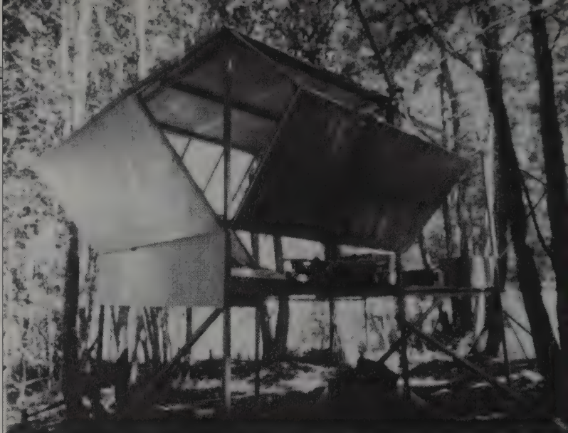
Even the temporary erecting crane of this portable house is Box Beam. The house has been moved several times, but has not yet been developed with sufficient detail to be a commercial venture.
